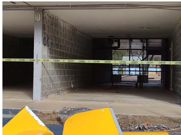
Flood water line ---->
